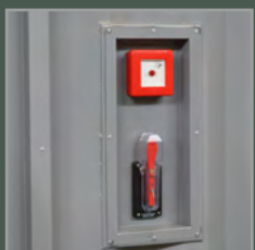
Emergency button lever to stop the oil and EPO
