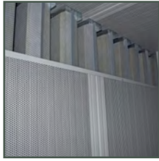
Air intake louvres and special attenuators for acoustic insulation
