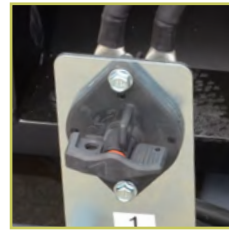
Battery isolator lockable, it is used during maintenance and storage
